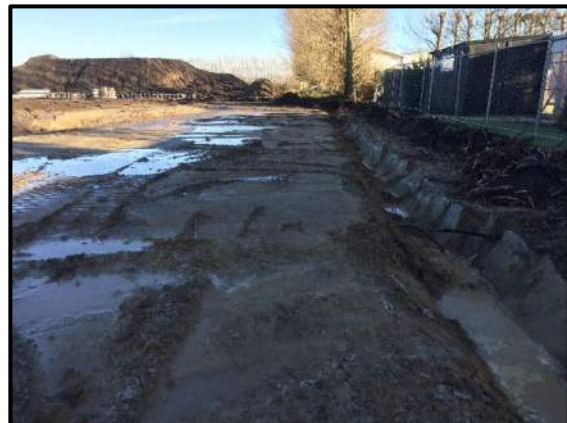
Photo 14: Service trench excavated on the northern perimeter of the right-of-way. Photo facing west.
