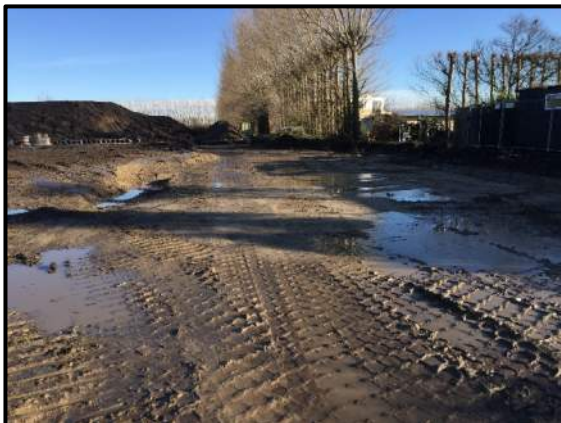
Photo 13: Lots 35 and 36. Note standing water in the base of the excavation. Photo facing west.
