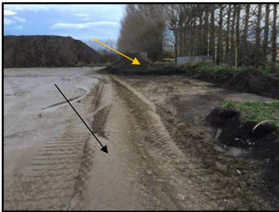
Photo 1: Within Lots 22 to 36 the upper 200 mm of the subgrade has been turned and recompactd (black arrow). Organic soil and topsoil stock piles were observed (orange arrow). Photo facing west.
