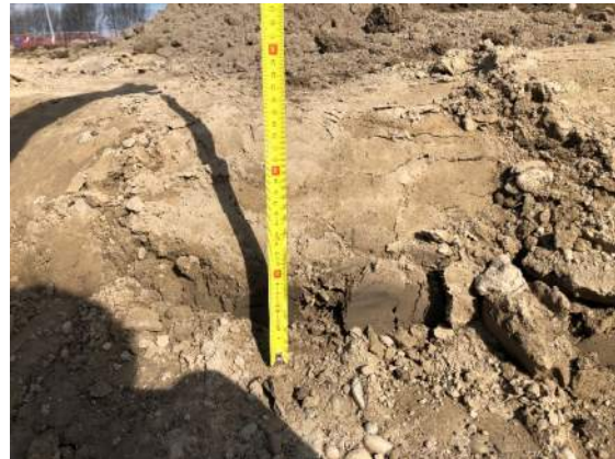
Photo 32: Depth of excavation below subgrade level to allow for backfill of pit run (subbase).
