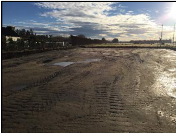
Photo 11: Lots 37 40 following placement of engineered fill. Note areas of saturated soil.
