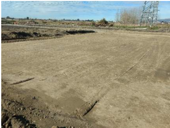
Photo 29: Lot 76 with the entire area over excavated and recompacted. Photo facing east.
