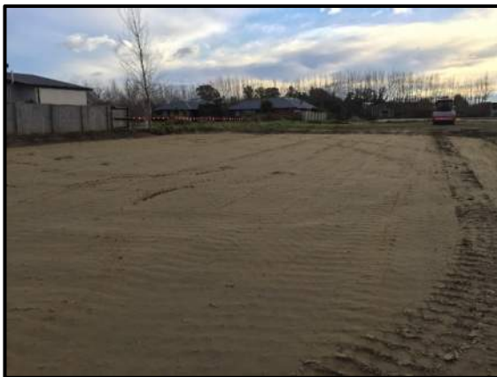
Photo 3: Lots 107 and 108 following compacted engineered fill suitable for topsoil placement. Photo facing north.
