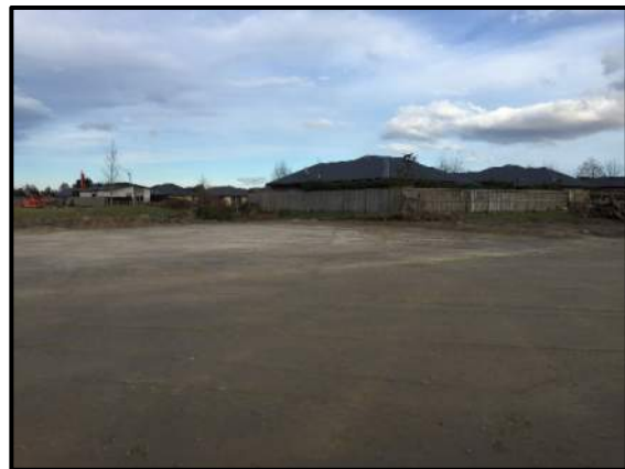
Photo 4: Lots 103 and 104 following compacted engineered fill suitable for topsoil placement. Photo facing west.
