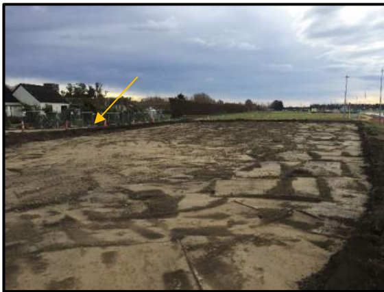
Photo 9: View of Lots 37 to 40. Right of way to be over excavated observed (orange arrow). Photo facing north.
