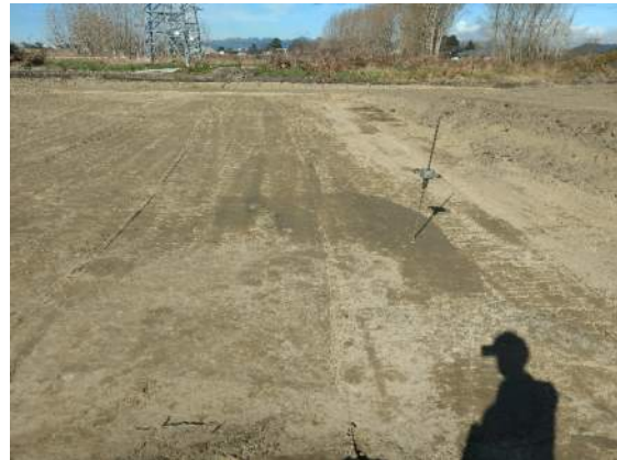
Photo 30: Lot 76 with the entire area over excavated and recompacted. Photo facing southeast.
