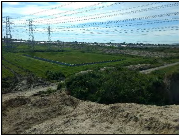
Photo 3: Silt, fill and unknown material stockpiles observed in Stages 1C, 5A, 5B and 5C of the development. Row of electrical tower pylons with adjacent stormwater retention basins observed.
